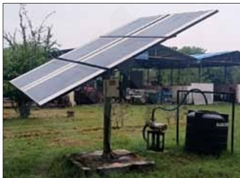
Fig. 10 : Solar pumping system
