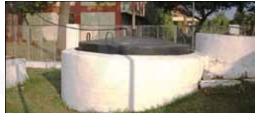
Fig. 5. Pile foundation based structurally modified floating drum type bio-gas plant for vertisols.
