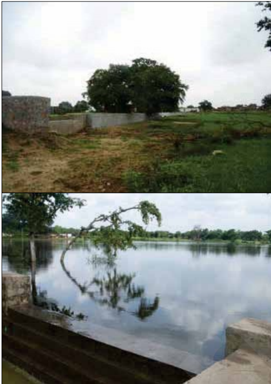
Fig. 3. Haveli renovation in Parasai-Sindh watershed; Masonry drop spillway (rectangular weir) and embankment along with corewall was constructed in 50 m breached area. Water harvested in Haveli during the monsoon period. Source: ICAR-Central Agroforestry Research Institute, Jhansi
