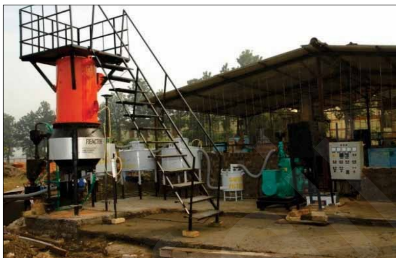
Fig. 4. A crop residue based electricity generation plant
