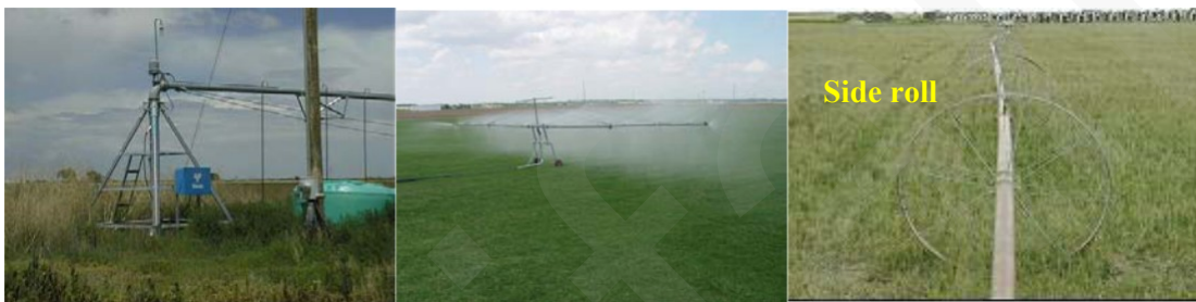
Fig .1 Example of a few rotating type sprinkler irrigation systems
